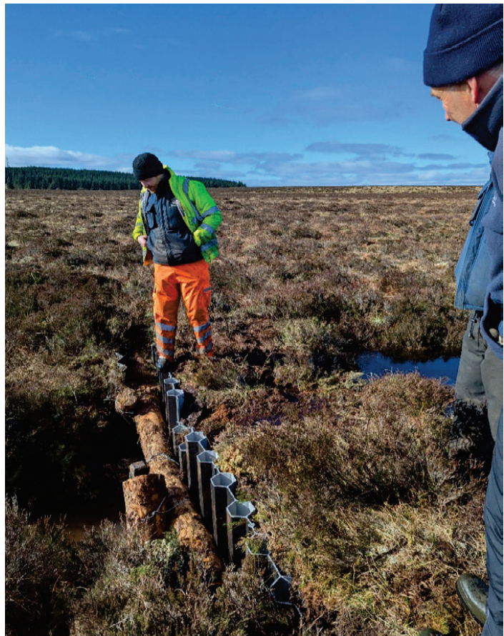
• Figure 9: Altikeeragh - hexagonal peat dam with log backup.
